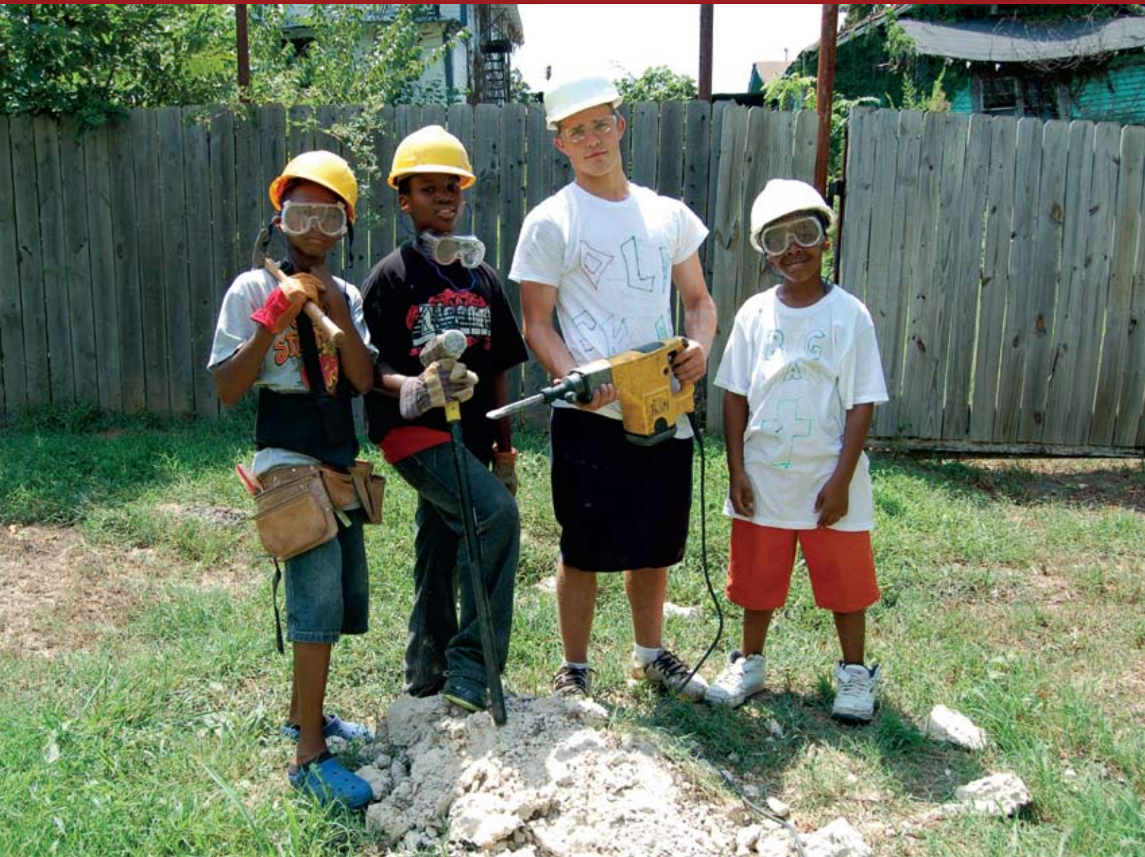
From left, Courtney, Treshawn, Luke Olson and Shamareio chip away at a patch of unwanted concrete in Allendale.
